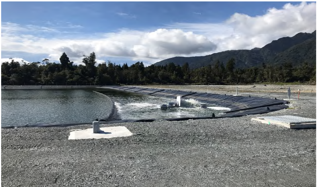
Aeration operational on the new pond No.1
